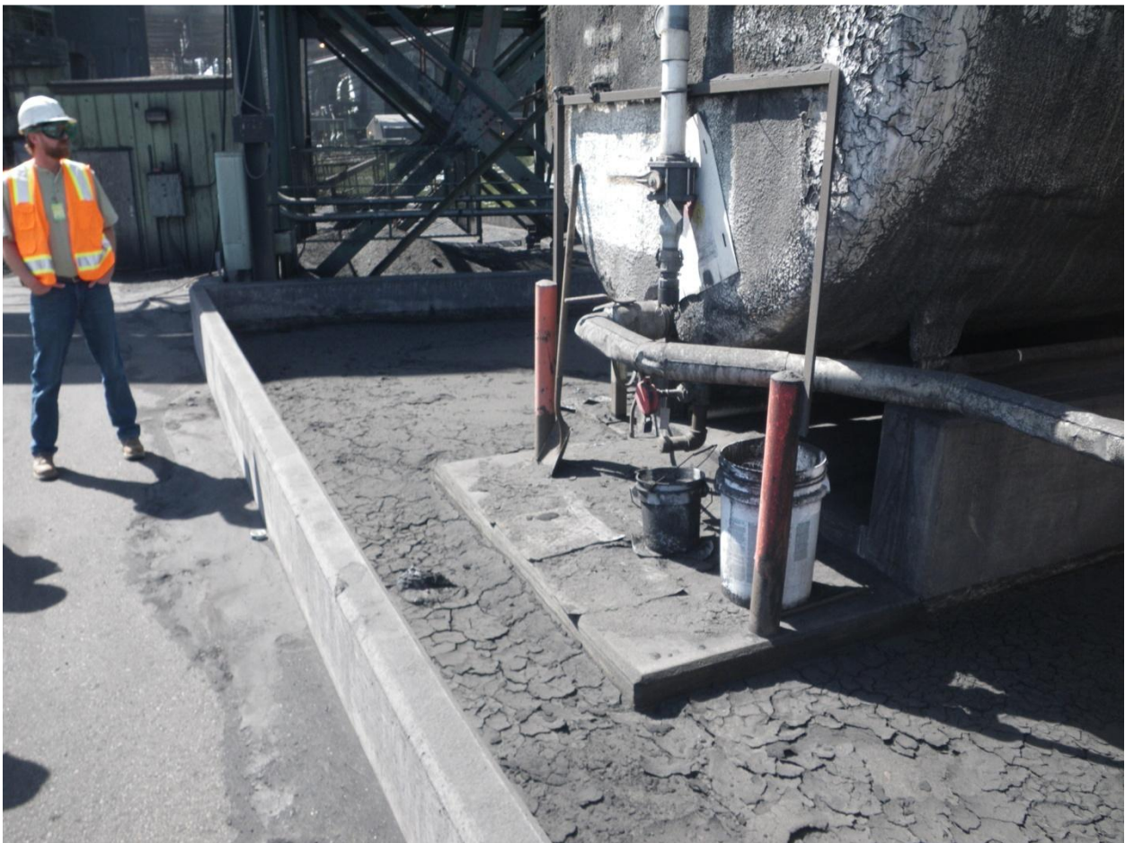
Figure 3: Flocculant for sump with containment. Ash build-up prevalent on the premises.
