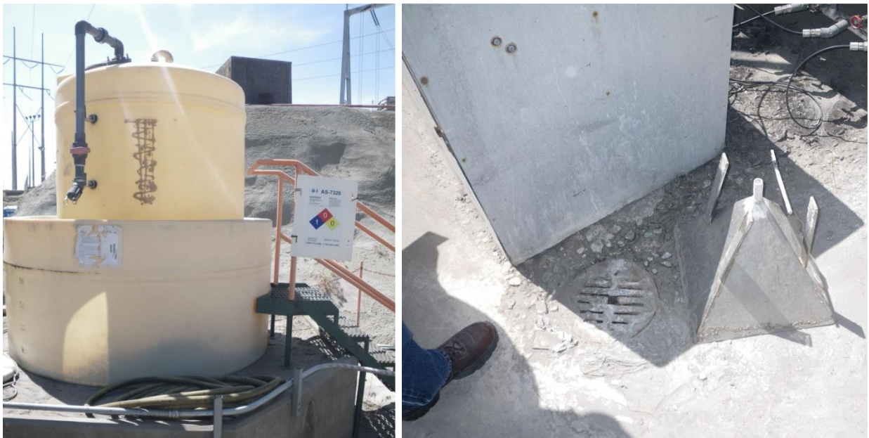
Figure 11: Corrosion inhibitor, acrylate copolymer (left) and chlorine powder addition (right).
